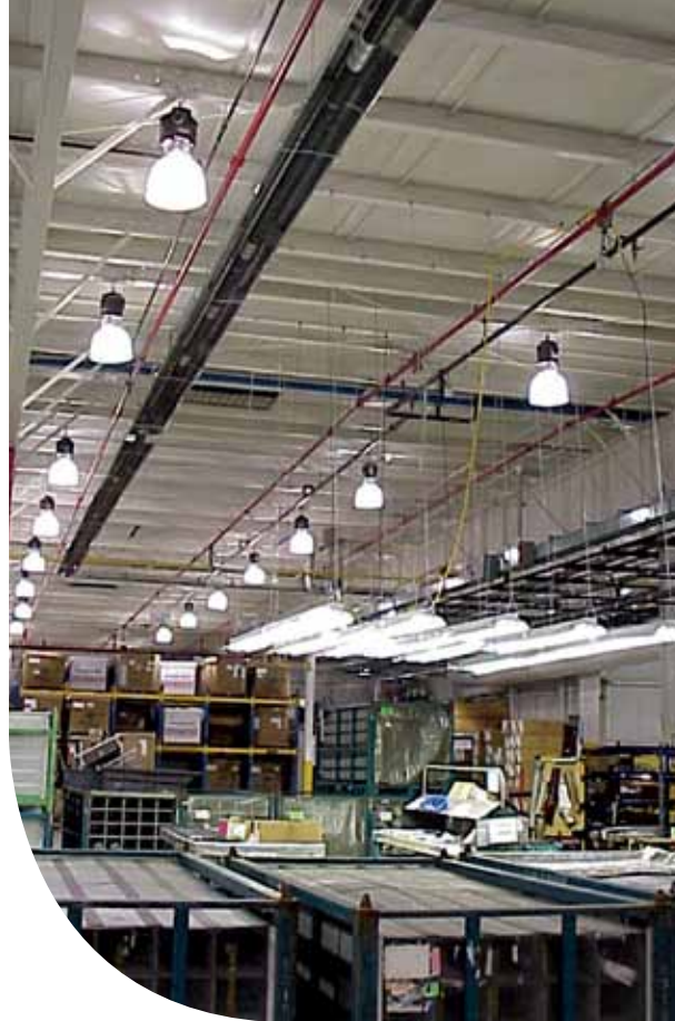
Workstations heated with infrared heaters.
