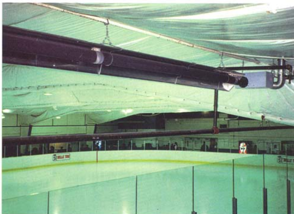
A low-intensity Tube Heater over bleachers at 30° angle at rink in Fraser, MI
